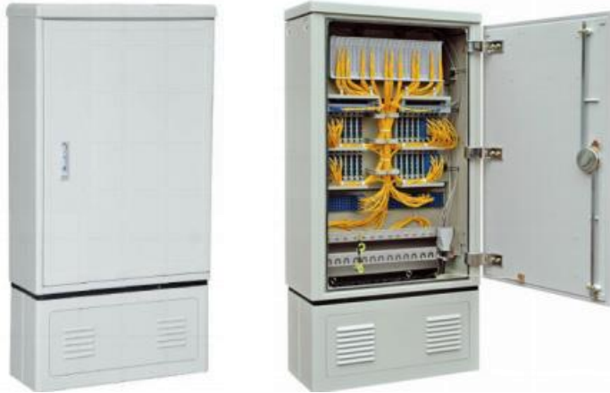
Optical Splitter Cabinet
